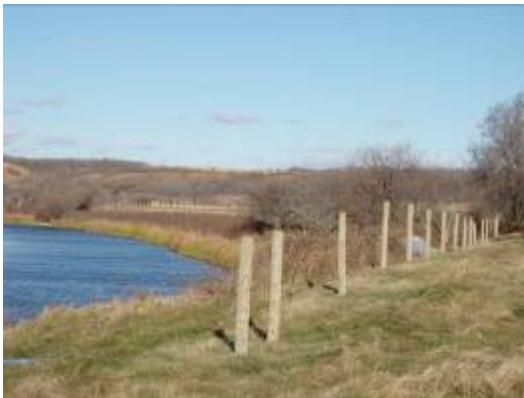
Installation of livestock exclusion fencing in the Little Saskatchewan River Conservation District. Photo: L. Remillard. © Environment Canada 2011.
