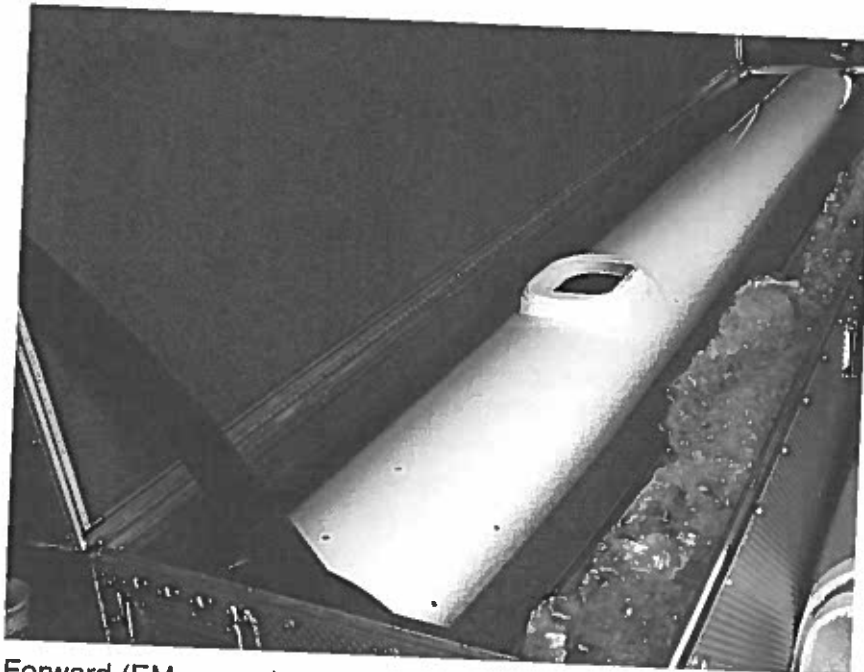
Installation on a Great Slave Helicopters 206L-4, looking forward, showing installation on the port side of the aircraft necessitated by the presence of a high-pressure nitrogen line on the starboard side.
